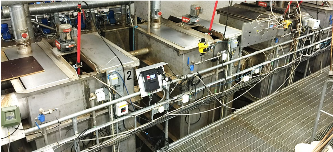
Figure 5. Photo of the top of biological treatment tanks BR2-4
