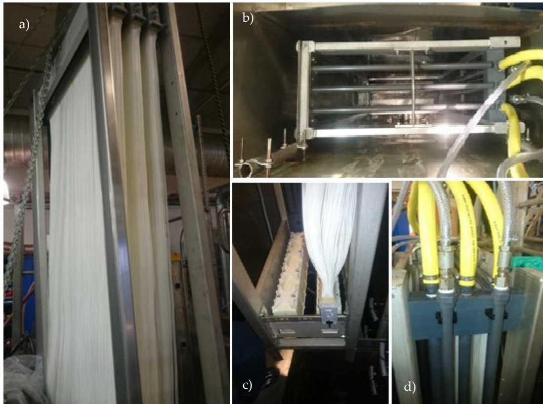
Figure 6. The membrane during installation of the pilot. a) Membrane cassette with three membrane modules, b) cassette lowered into the tank, view from above, c) mounting and aeration equipment at the bottom of the cassette, d) permeate connections (yellow) at the top of the cassette.
