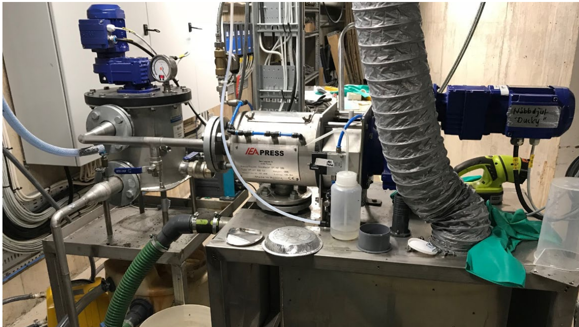
Figure 9. Photo of the dewatering equipment in the pilot.
