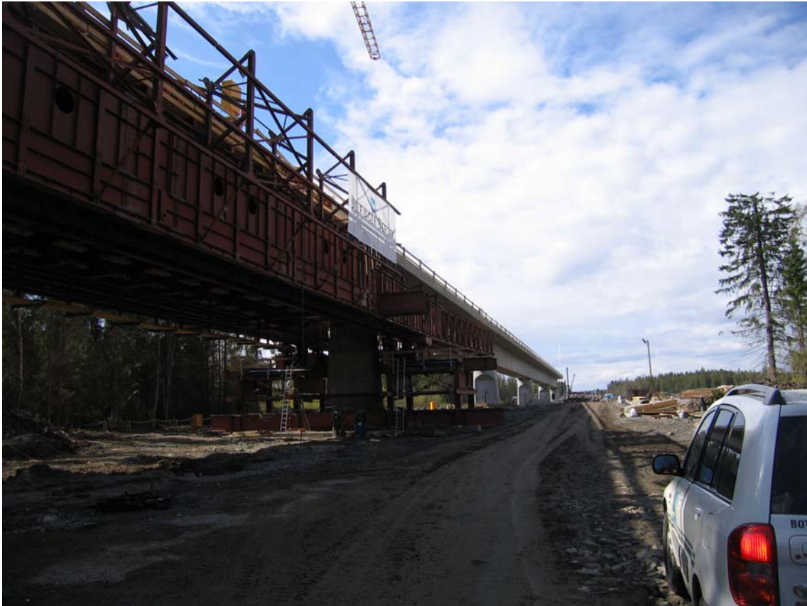
Figure 19 A concrete beam railway bridge under construction. The slipform is shown in the foreground and the finished bridge is shown in the background.
