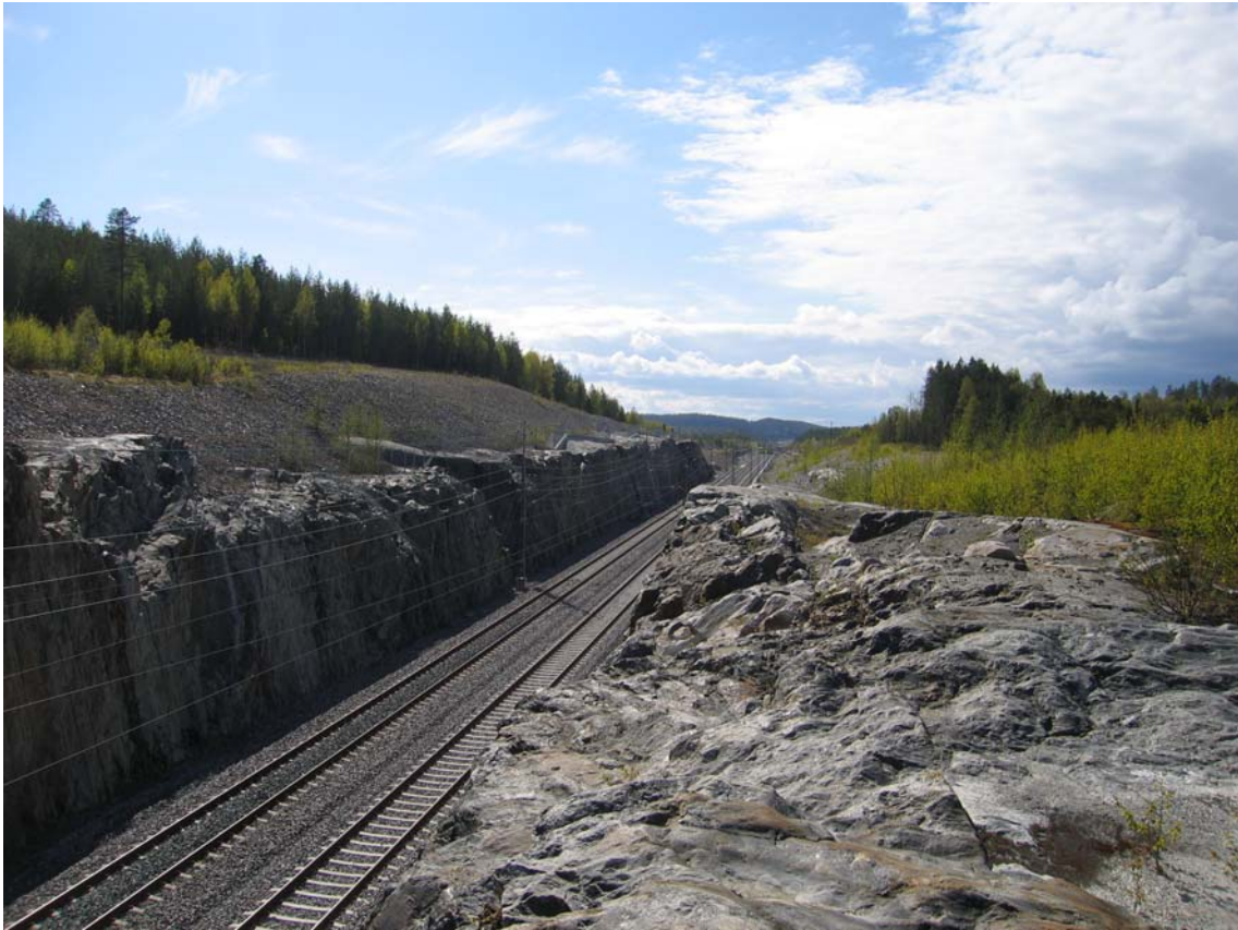
Figure 9 The railway track do not usually follow the landscape. In this case, excavations are needed. This picture shows an example of a hard rock excavation (a rock cutting).
