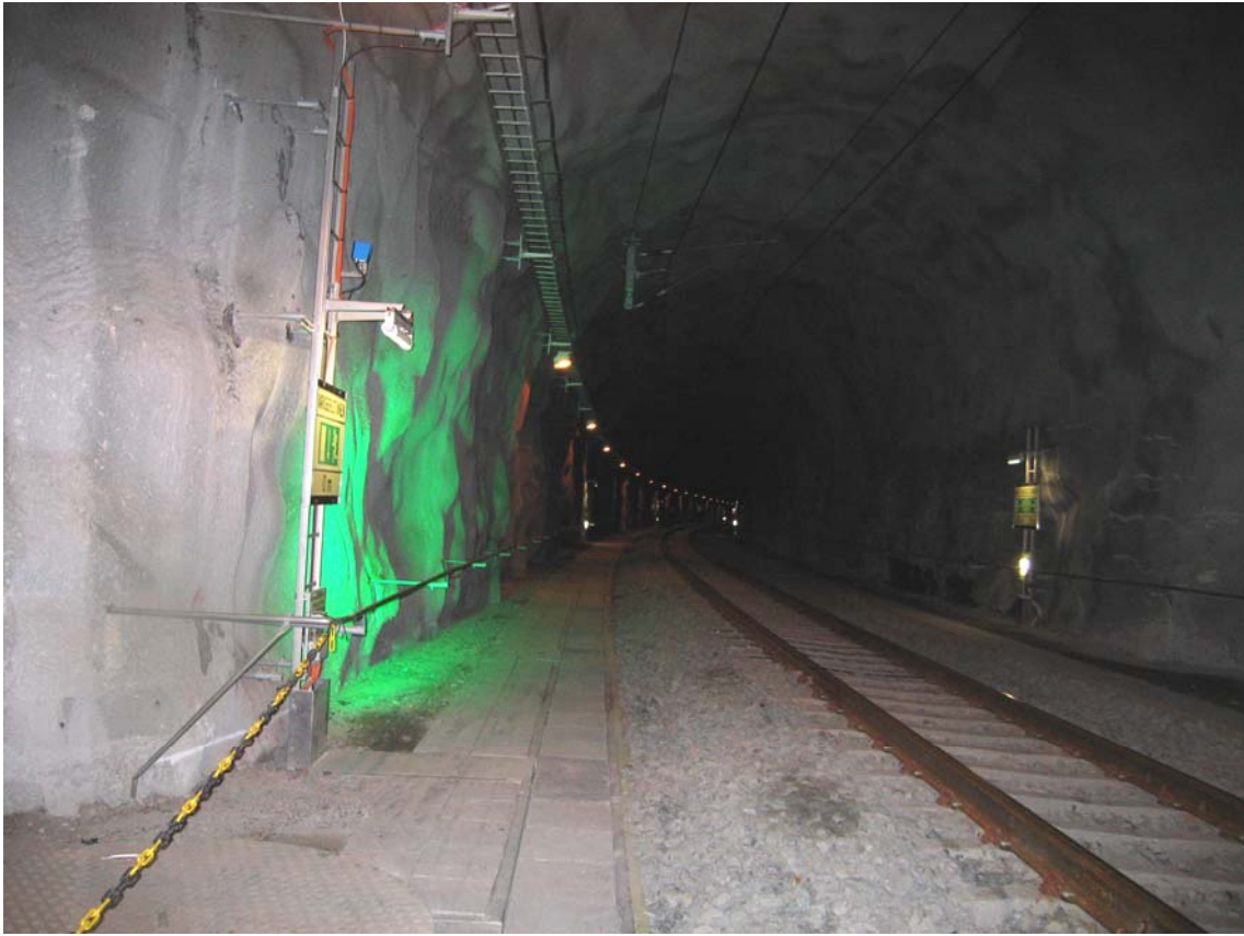
Figure 15 The picture shows an example of a main tunnel (train tunnel) with the different equipments.
