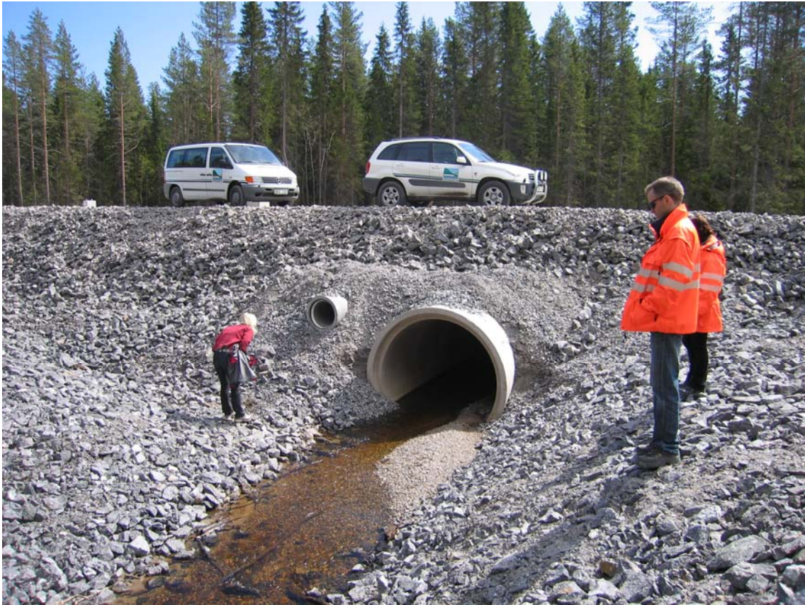
Figure 8 Culverts are needed in the track foundation for water and wildlife. The picture shows a culvert for a water course (large) and a separate, dry wildlife passage (small).
