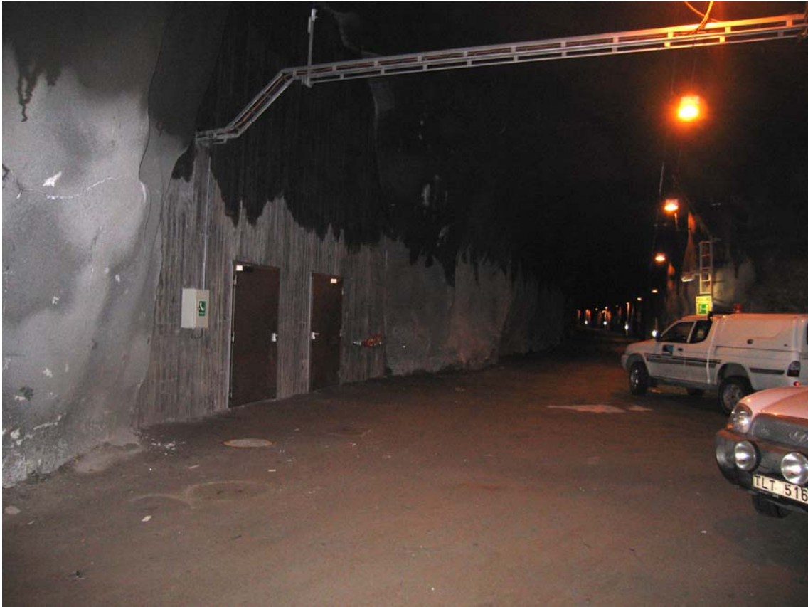
Figure 16 Example of a service tunnel. The doors are a part of the evacuation lock from the main tunnel to the service tunnel.
