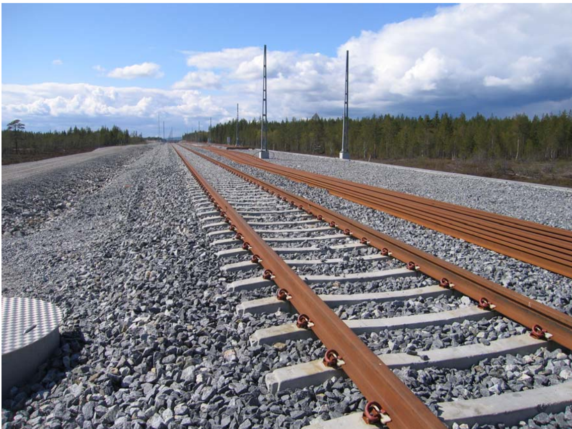
Figure 10 The picture shows a typical railway track with rails attached to concrete sleepers with rail fastening. The space between sleepers are filled with track ballast.
