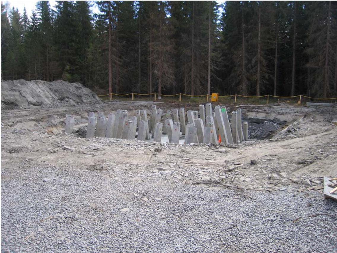
Figure 20 The picture shows an example of foundation work for a bridge pier. In this case, the ground has been excavated, stabilized by precast concrete piles and a concrete foundation has been cast.
