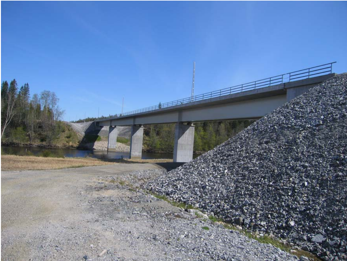
Figure 18 A steel girder railway bridge. To the right in the picture, the erosion protection of the slope is shown.
