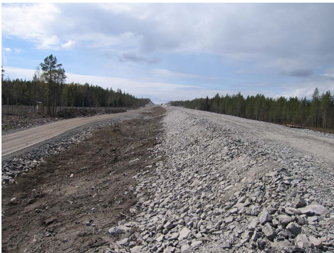
Figure 7 To the right, a typical railway track foundation. The service road parallel to the railway is shown to the left.
