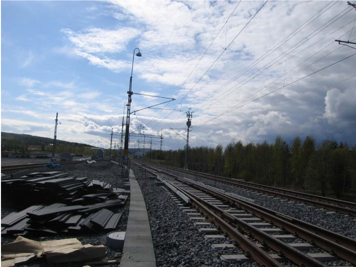
Figure 11 The picture shows power supply line for train operation. On the pole to the right a pole transformer is shown.
