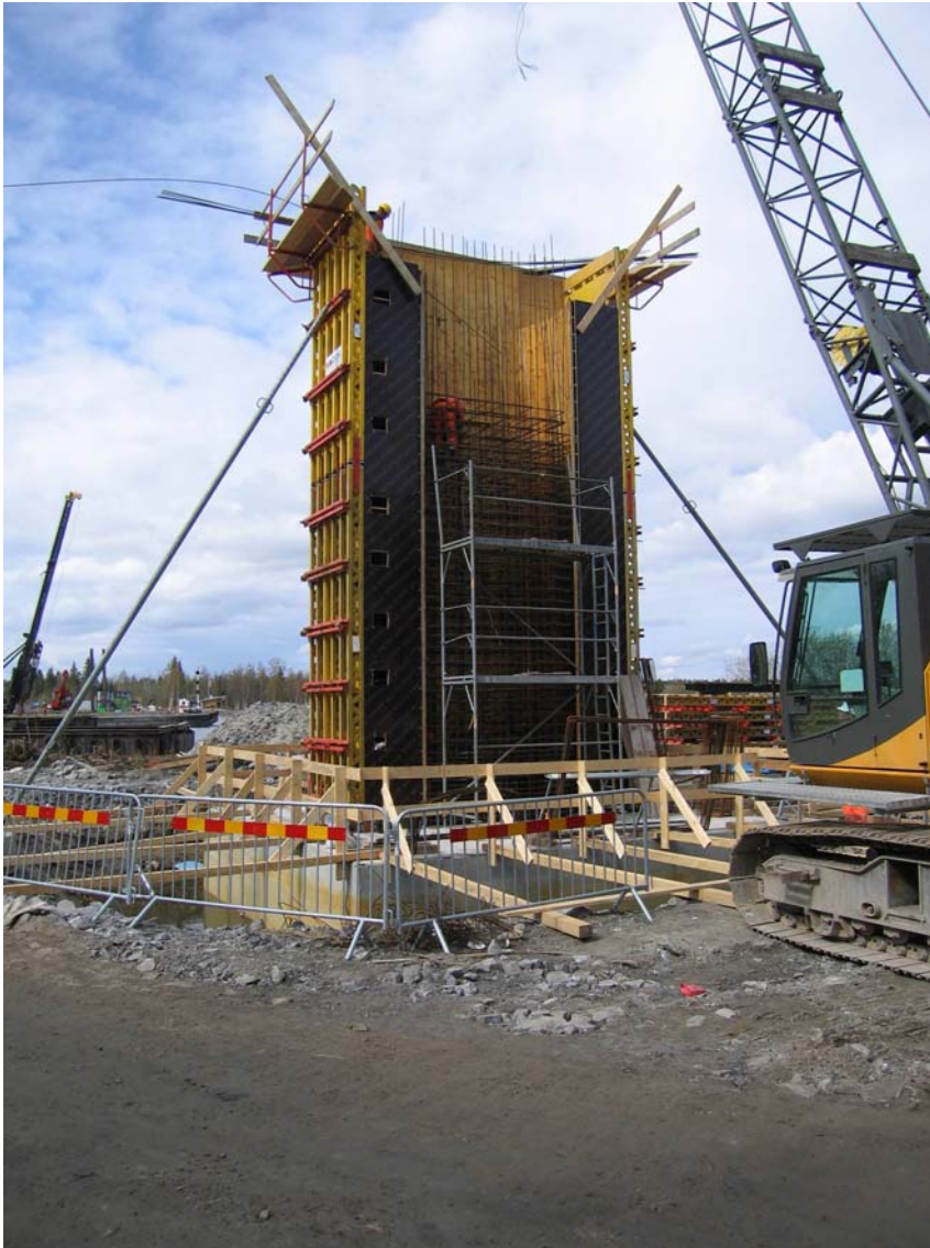
Figure 21 Casting of a railway bridge pier on top of the foundation. In the picture, the concrete mould with the steel reinforcement is shown.
