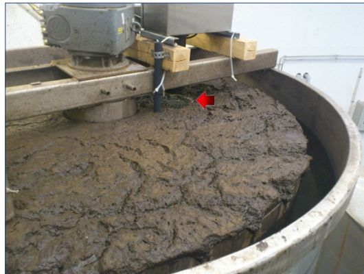
Figure 14. Sedimentation basin with thick top sludge layer and visible dilution near the sensor that is generated by the automatic cleaning of the CBX sensor.
