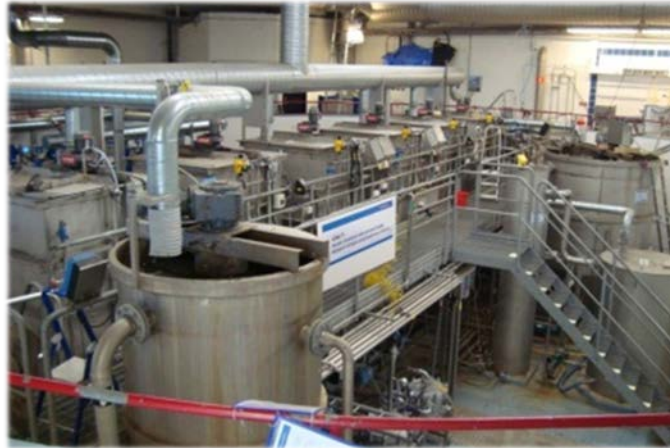
Figure 10. Line 1 of Hammarby Sjöstadsverk that was used in this test. Line 1 was operated as a conventional WWTP with chemical phosphorous removal.
